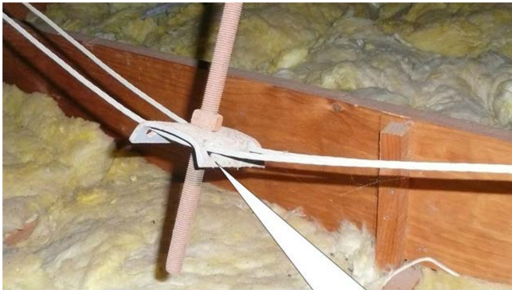
Example of the tensioning mechanism – the roof carpenter simply screws down the nut to tension the pair of cables
