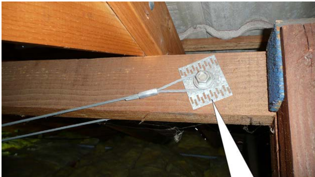
Example of the connection point for the cables
